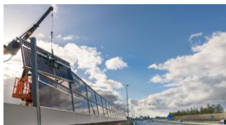
Infrastructure-integrated PV (IIPV)
